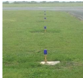
Figure 2: Taxiway Edge Lights
